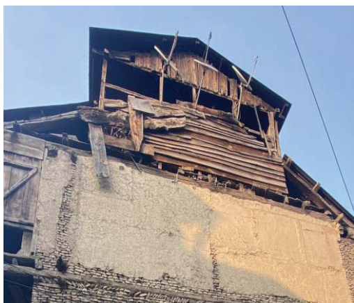
(a) Deteriorated timber
