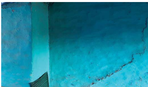
(a) Crack in walls
