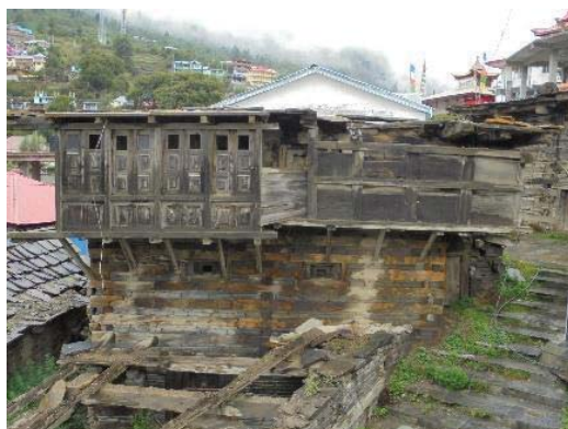
(a) Deteriorated building
