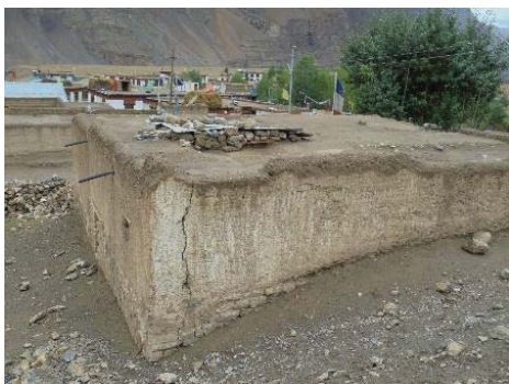
(a) Deteriorated building
