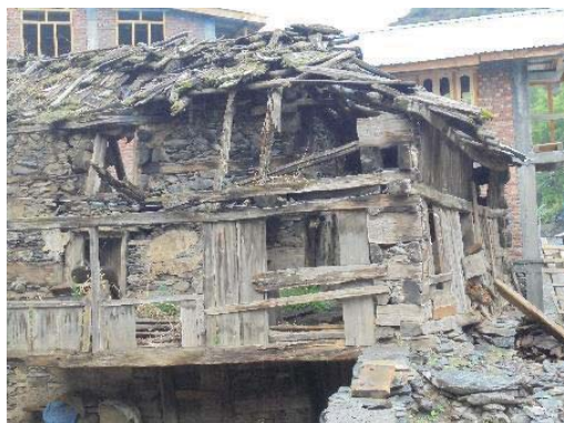
(a) Deteriorated building
