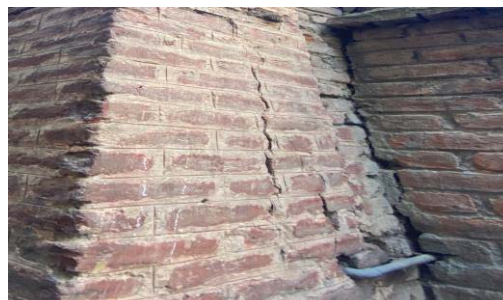
(b) Crack in walls
