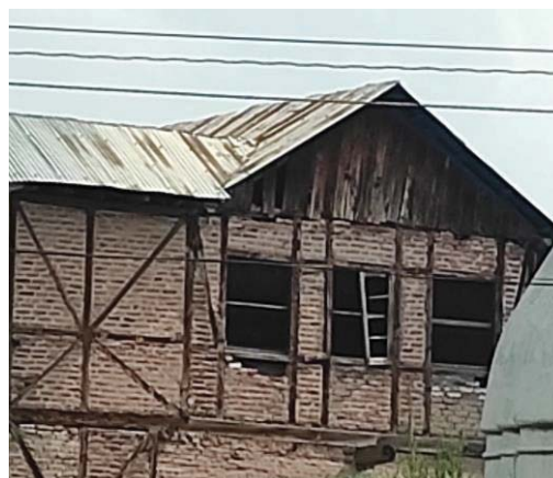
(b) Damaged infill walls
