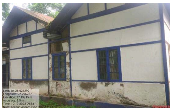
(b) Plaster deterioration
