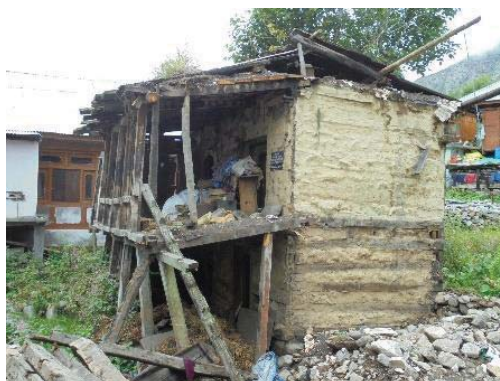
(b) Deteriorated building
