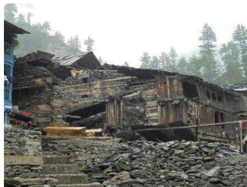
(b) Deteriorated building
