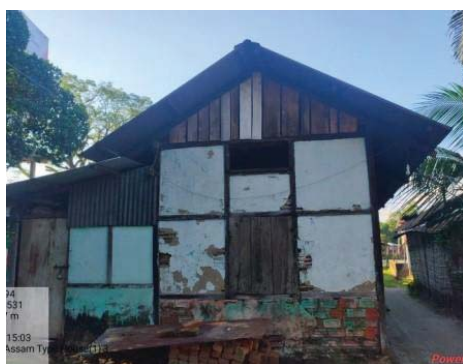
(a) Plaster deterioration
