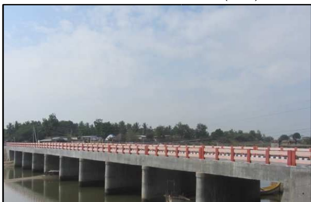
Bridge in km 2/4 of Bapatla Pandurangapuram road in Guntur District, (A. P.)
