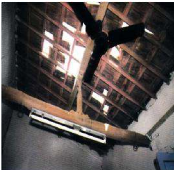
Damage primarily caused by strong winds
