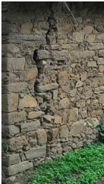
Separation of the wall from stone pier
