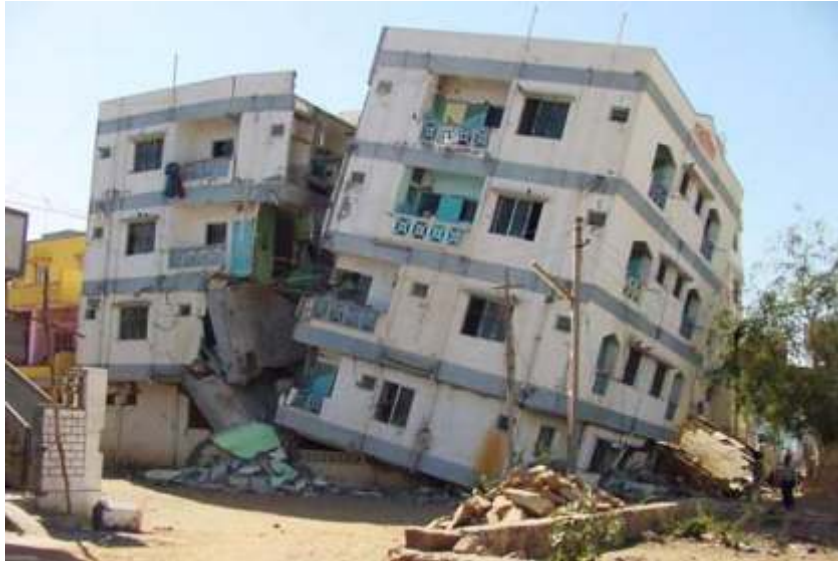
Collapse of reinforced concrete columns (and building) during 2001 Bhuj (India) earthquake
