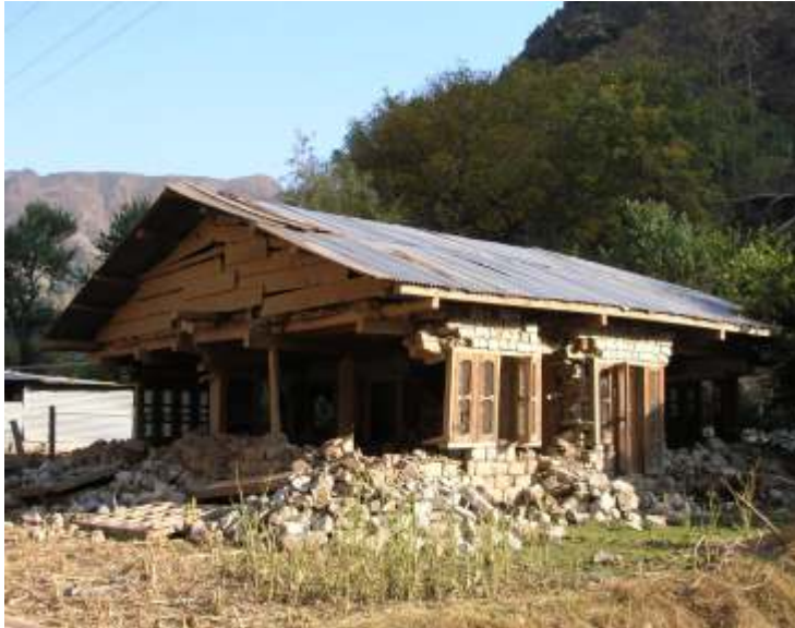
Out-of-plane damage to the exterior wall.
