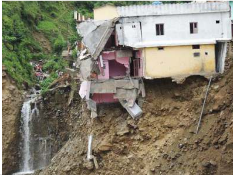
Damage to sub-structure
