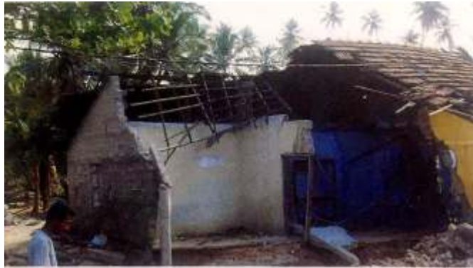
Damage due to strong winds
