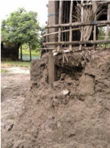
Scouring of foundation
