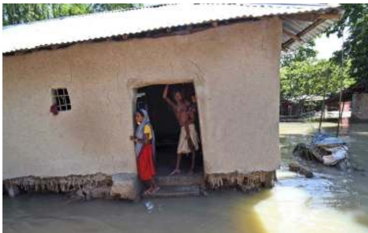
Settlement of foundation.
