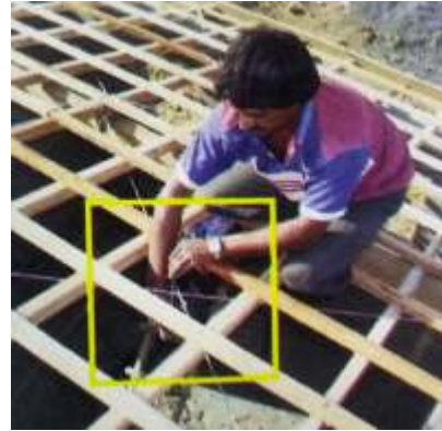
Pre-tension wires by twisting all wires along one diagonal together with a piece of rebar.
