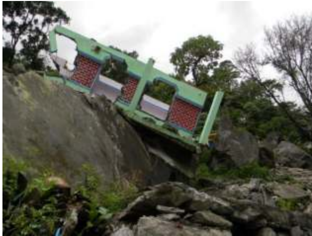
C3 Hazards: Their Severity, Zonation and Impact on buildings NDMA Unnati PIC
