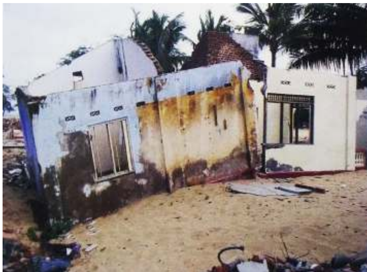
Damage due to foundation settlement
