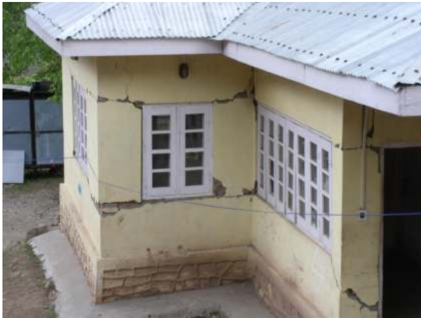
Diagonal cracks around openings
