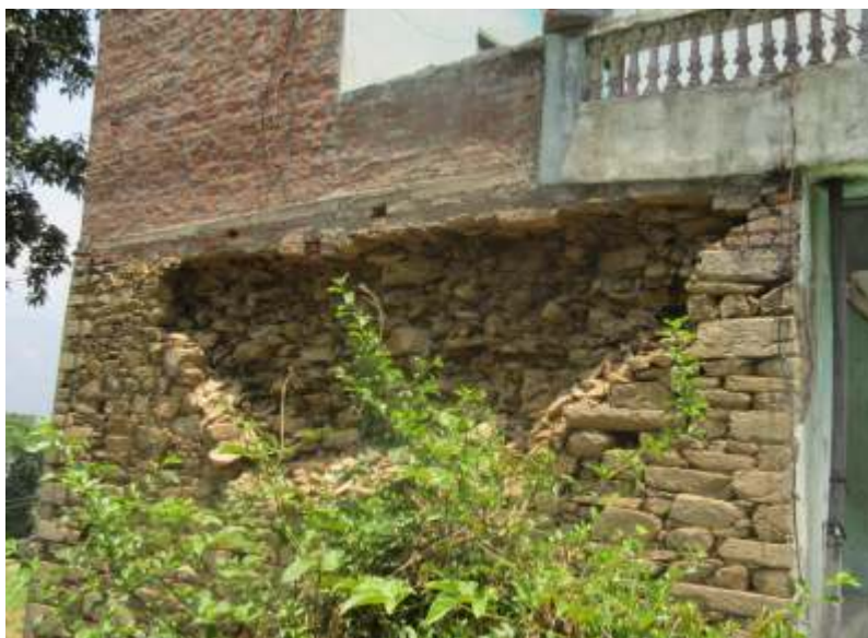
Delamination of stone wall
