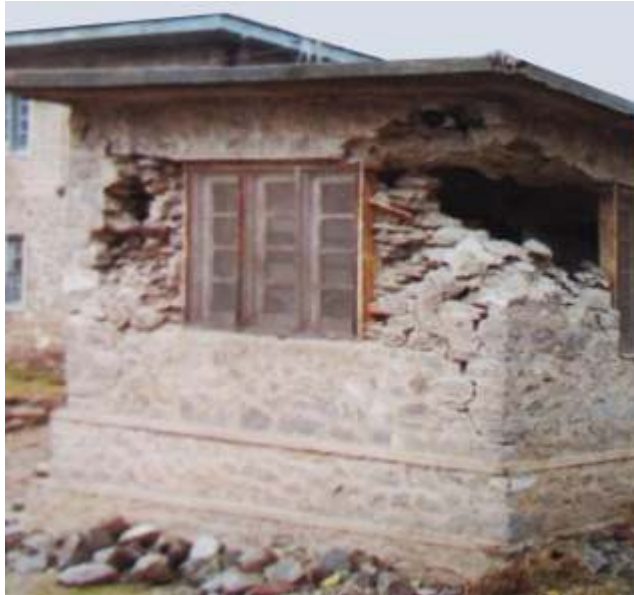
Damage at the corners of the house.
