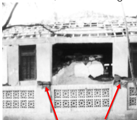
Masonry piers cracking
