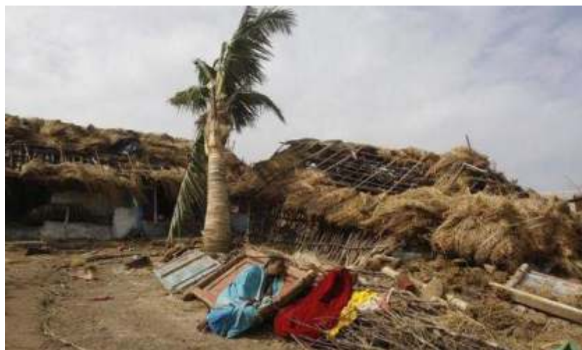
Severe damage to load bearing structures
