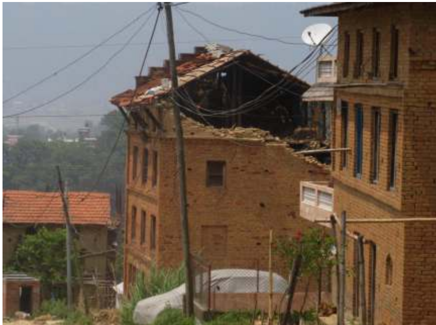
Collapse of the gable wall.
