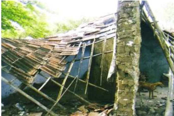
Damage to roof structure
