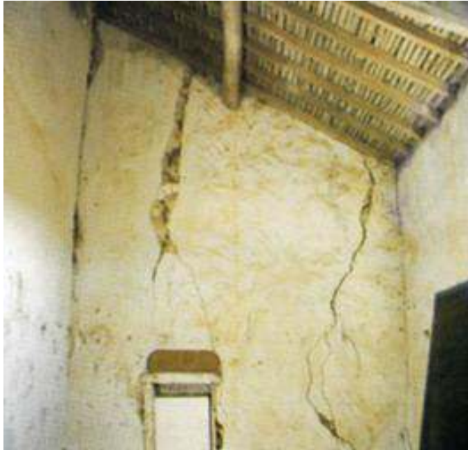
Cracks on the gable wall.
