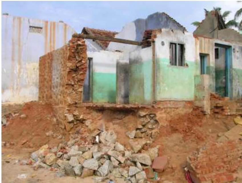
Damage to the substructure and super-structure
