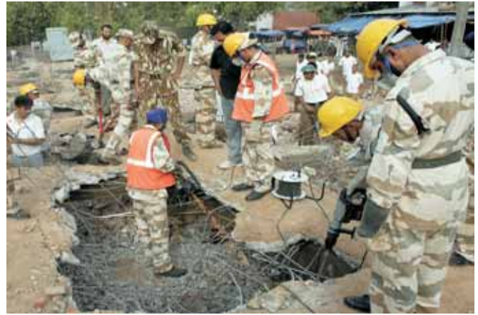
NDRF at the site of roof collapse at subzi mandi , Chandigarh
