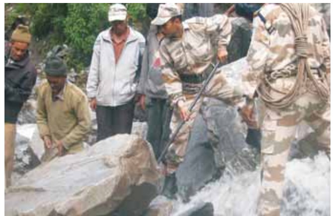
SAR team clearing a landslide near Amarnath (J&K)
