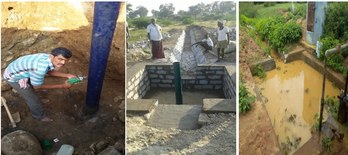
Figure 5.2: Injection & Recharge Well
