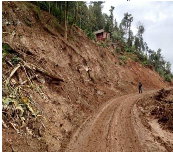
Close view of a Debris slide occurred along Hirebail-Hemmakki road at Malleshwaragudda.
