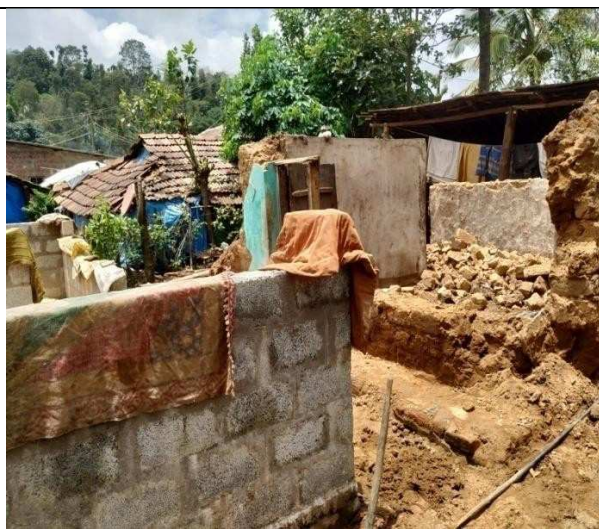
Construction of house at the flood plain area with weak basement
