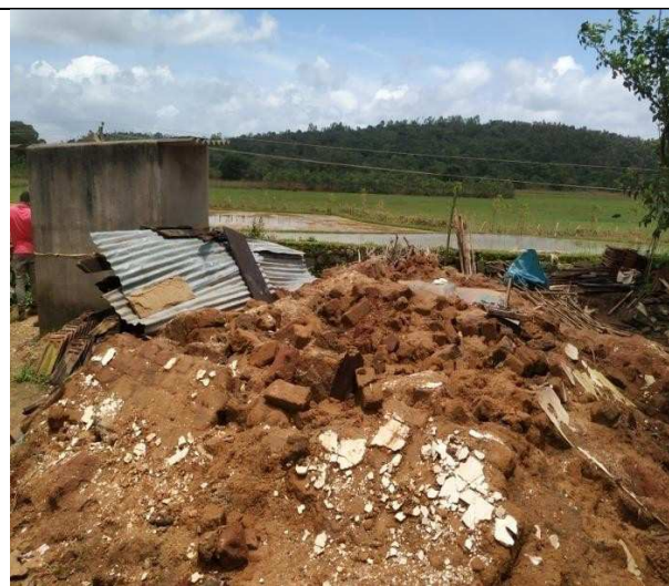
Completely collapsed house due o flash flood
