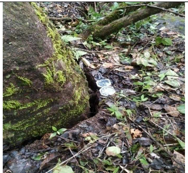
Crack is formed at the contact of rock and soil
