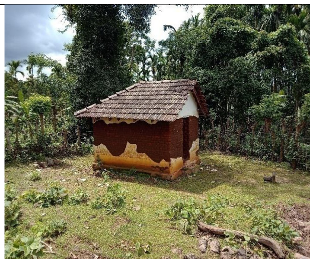
Damaged house due to flooding
