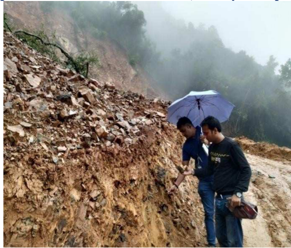
Highly weathered and thickly saturated mass contributing the weight on slope
