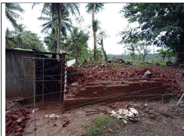
Damaged house due to flooding
