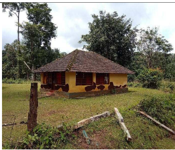
Damaged house due to flooding
