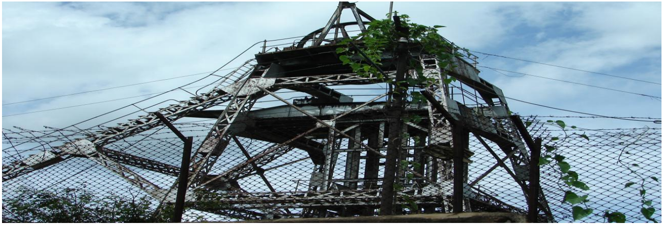
Dilapidated Head shaft of BGML
